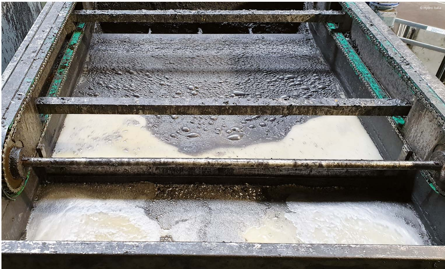
The Hydrofloty 24M sludge separation system.
